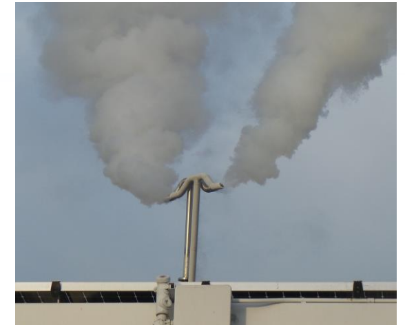
Venting very cold hydrogen initially horizontally at the Emeryville H 2 Station, Emeryville CA.
